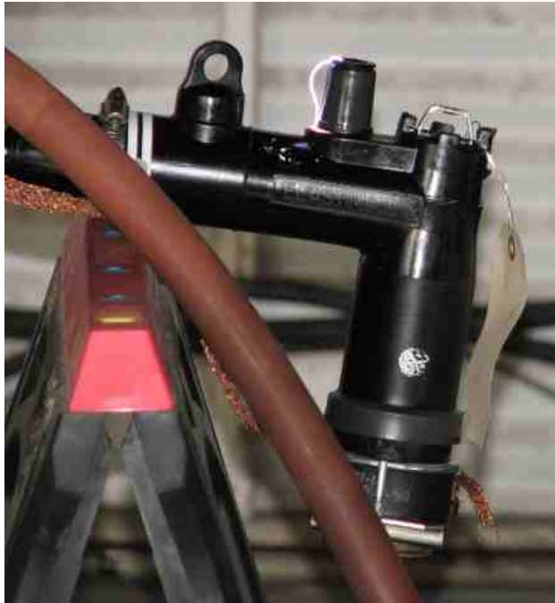
Figure 4: Flashover during high voltage test.
